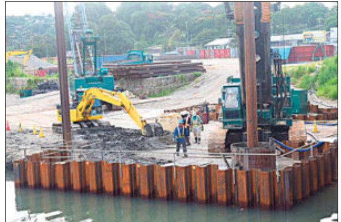
Construction work underway at Mataniko bridge, Central Honiara, will relieve the traffic chaos and reduce cost of doing business in the capital.
